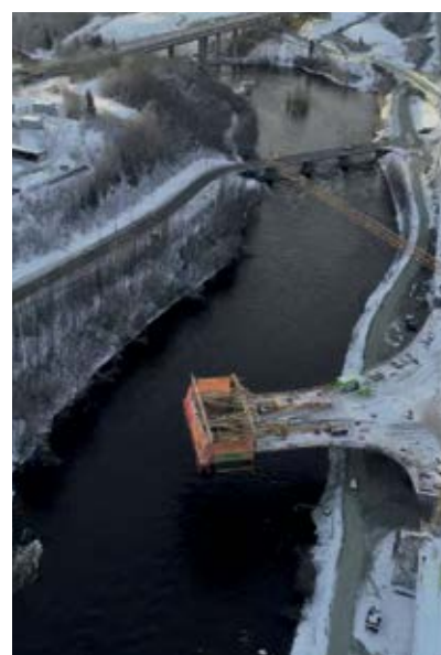
SKÅKABELBRU: Nydalsbrua is built according to the free-build method. The bridge is cast in eight different stages from the Byåsen side towards the Sluppen side, where each stage is 8.5 metres.
